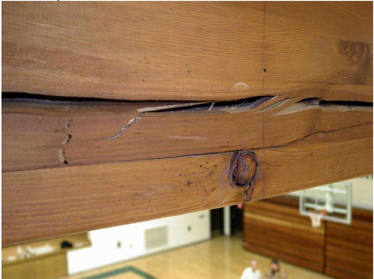
Figure 1. Failed beam due to overstress in bending.
