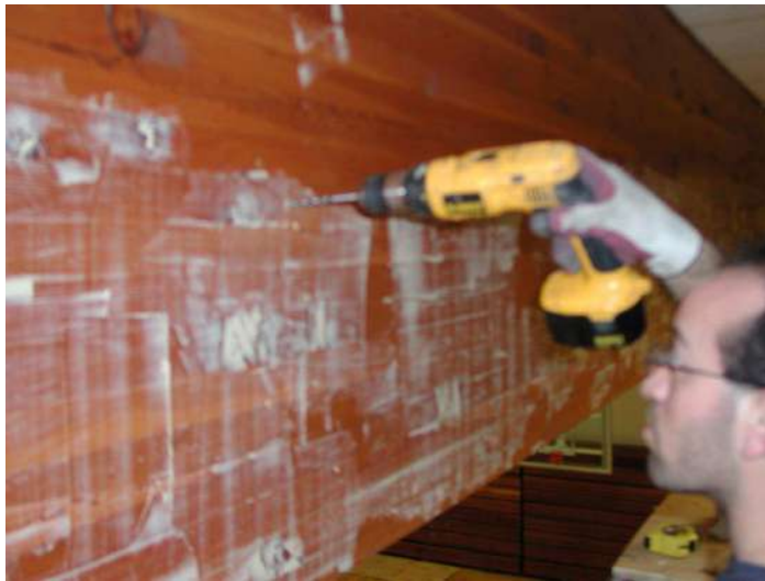
Figure 5. Drilling the injection and exhaust ports. Epoxy paste is used to seal the sides of the beam.
