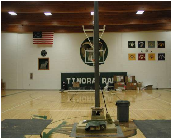
Figure 3. 152 x 152 HSS member used to jack beam to unloaded position during beam repair.
