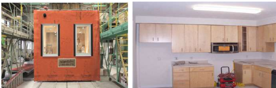
Figure 8. Window and cabinet installation in a module. (Image sources: Deluxe Building Systems)
