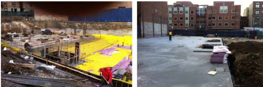
Figure 10. Conventional construction for the foundation and first floor slab. (Image sources: Deluxe Building Systems)
