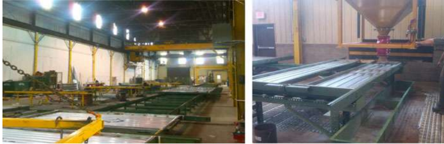
Figure 3. Steel slab frame and poured concrete on the slab form. (Courtesy of Deluxe Building System)
