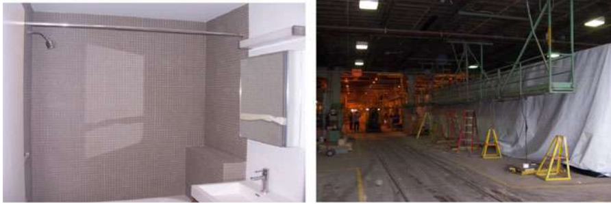
Figure 9. Tiling a bathroom and weatherproofing the module for transport. (Image sources: Deluxe Building Systems)
