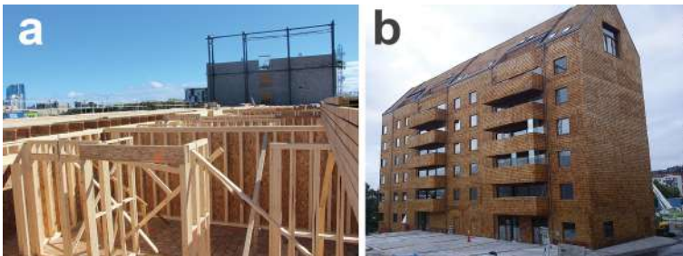
Figure 1.1 Residential buildings using a timber structure: (a) Light timber framed mid-rise building in Canada (photo Cecobois); (b) Residential building in Sweden (photo B. Östman).
