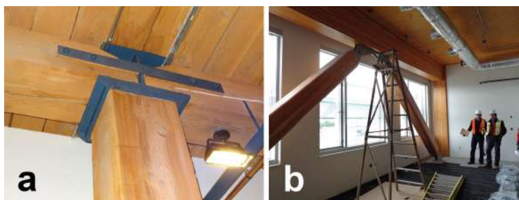
Figure 1.7 Post-and-beam timber constructions: (a) Old timber frame in Canada (Photo FPInnovations); (b) Modern post-and-beam construction using braced frames in Canada (Photo A. Buchanan).
